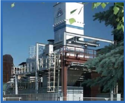
Gas-turbine electric power unit with the capacity of 2,5 MW
