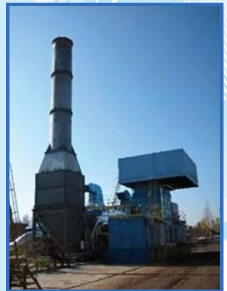
Gas-pumping unit at the Permskaya compressor station
