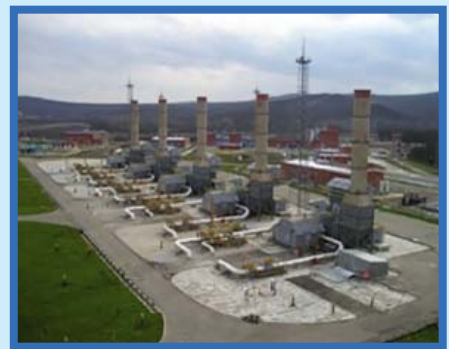
Gas-pumping unit with the capacity of 12 MW at the Krasnodarskaya compressor station
