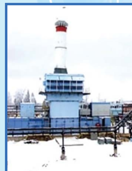
Gas-pumping unit for underground gas storages with capacity of 10 MW at the Karashurskaya compressor station
