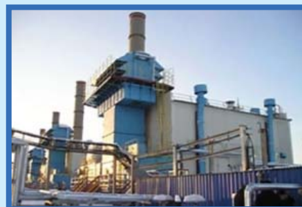
Booster gas-pumping unit with the capacity of 16 MW at the Zapadno-Tarkosalinskaya compressor station
