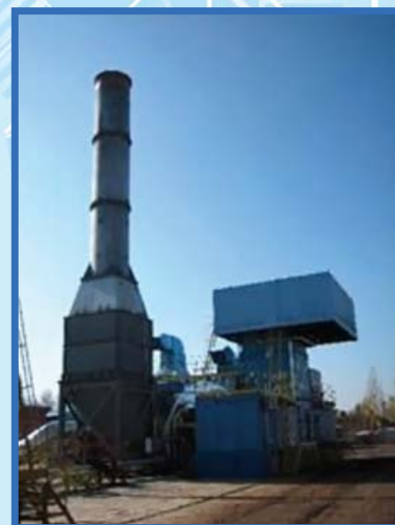
Gas-pumping unit at the Permskaya compressor station
