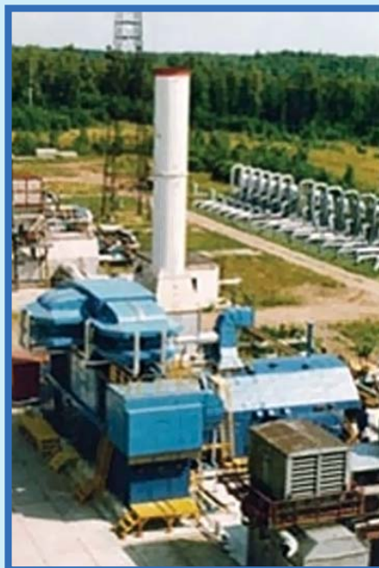
Gas-pumping unit consisting of self-contained assemblies with the capacity of 12 MW
