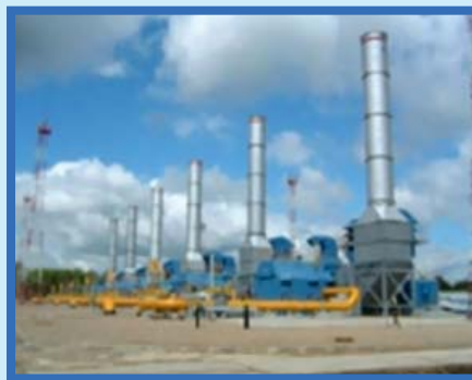
Gas-pumping unit with the capacity of 16 MW at the Smolenskaya compressor station
