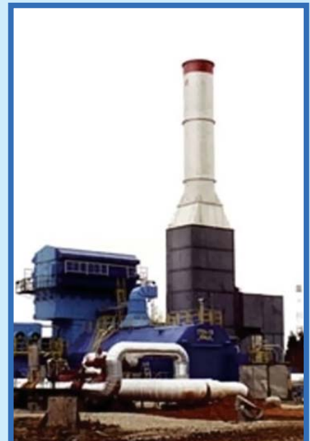
Gas-pumping unit with the capacity of 16 MW
