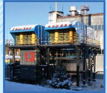
Gas-pumping unit at the Igrinskaya compressor station
