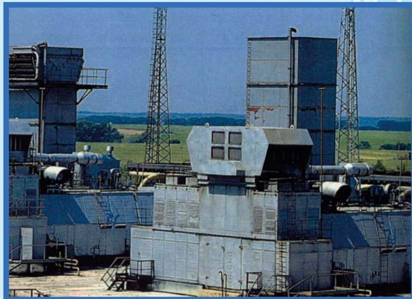
Gas-pumping unit based in the 8 MW engine
